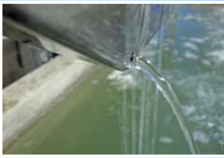
In the images; phosphate treatment which is also made to the inner parts of the hull.
